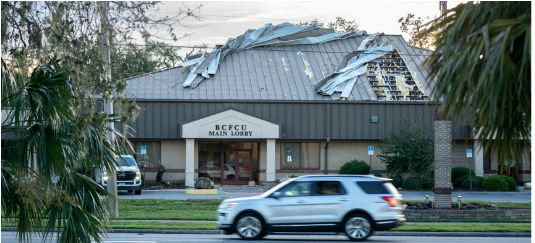
A building in Perry, Florida, with roof damage after Hurricane Idalia crossed the state on Aug. 30, 2023. SEAN RAYFORD/GETTY IMAGES
